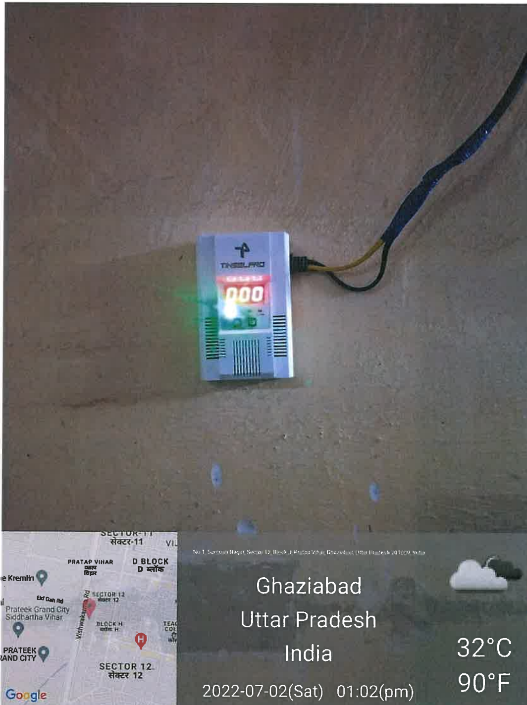
Gas Leakage Sensor System in Canteen
